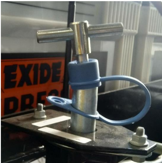
Battery cutoff Switch
