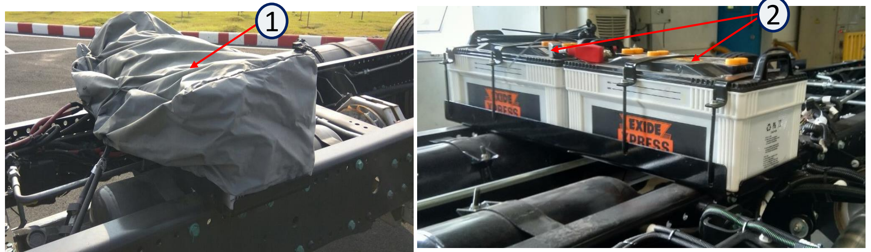
Battery compartment B54.10-0009-02 Electronic relays (arrows) 1 Plastic cover for battery protection 2 Protection removed from batteries
