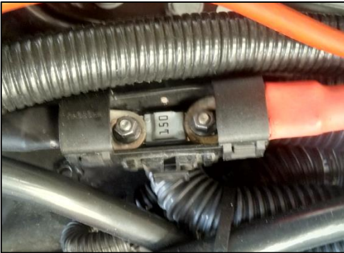
Retarder Power supply fuse (1x150A)
